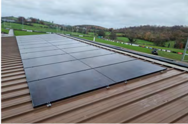
Traugh Gaels GFC- Solar PV System
