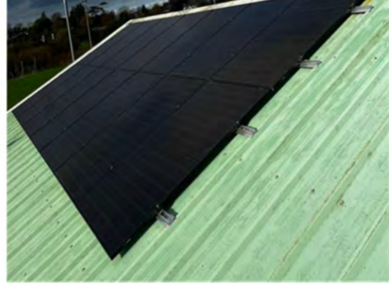
Cremartin GAA- Solar PV System
