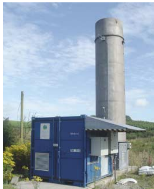
Changes to landfill gas flare motor resulted in energy savings.
