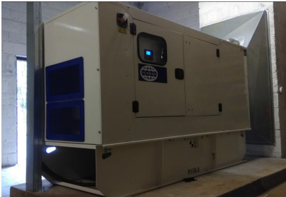
Generator installed in Head Offices at the Glen
