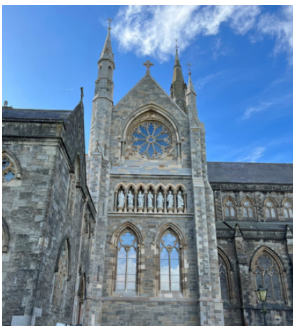
Repaired Windows, Stonework, Leadwork and Flashing to the North Transept Gable of Monaghan Cathedral
