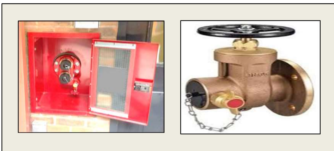
Figure 11(a) Inlet Breeching at exterior of building
