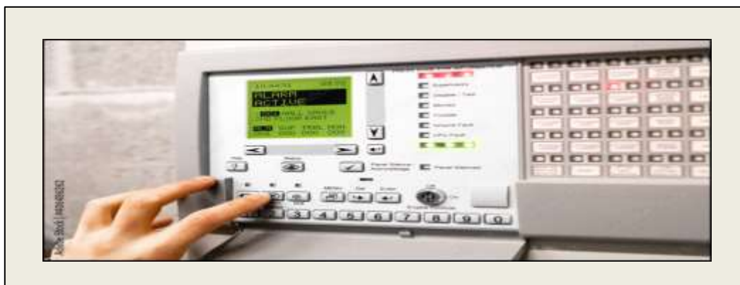
Figure 5 Fire Alarm Panel
