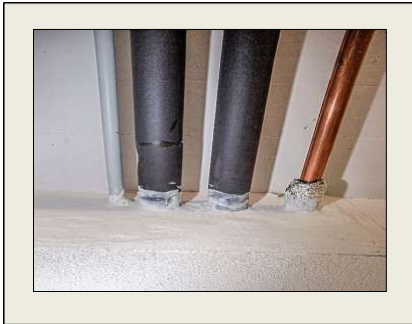
Figure 20 Fire Stopping of Pipe Penetration Wall
