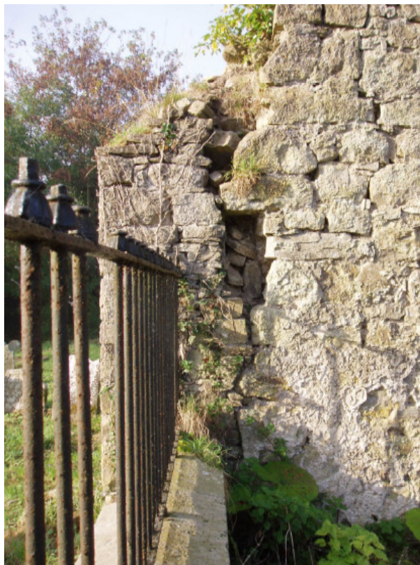
Fig. 10 Close-up of the severe crack in the east-facing elevation of the west gable of the church. The detached end of the wall needs to be pinned back to the main panel of masonry and the void infilled
