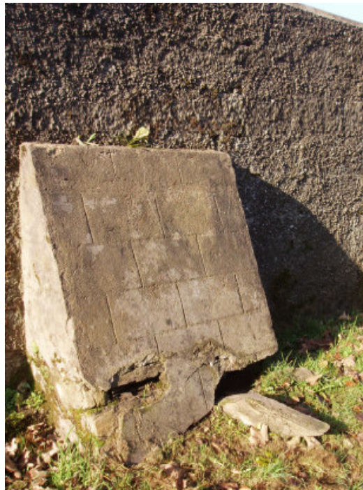
Fig. 42 Detail of the buttress which requires attention. An inspection of the existing walls foundations should be undertaken prior to specifying what actions regarding any future buttressing works to the wall are required
