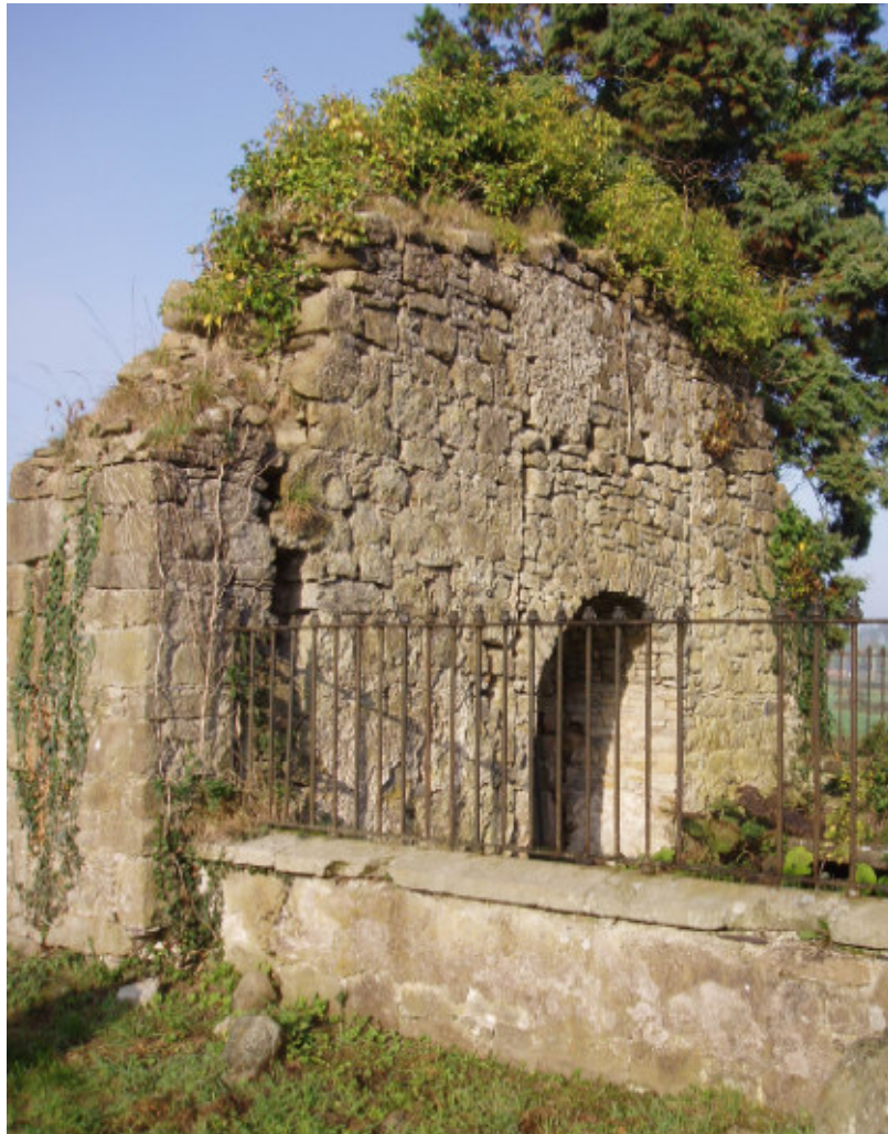
Fig. 8 The east-facing elevation of the west gable. The large crack in the foreground has resulted in the end of the wall becoming detached from the main panel of masonry. We would suggest that the end of the wall be pinned back to the main panel and the void infilled. The vegetative growth along the top of the wall requires removal and any loose capping stones discovered re-bedded.
