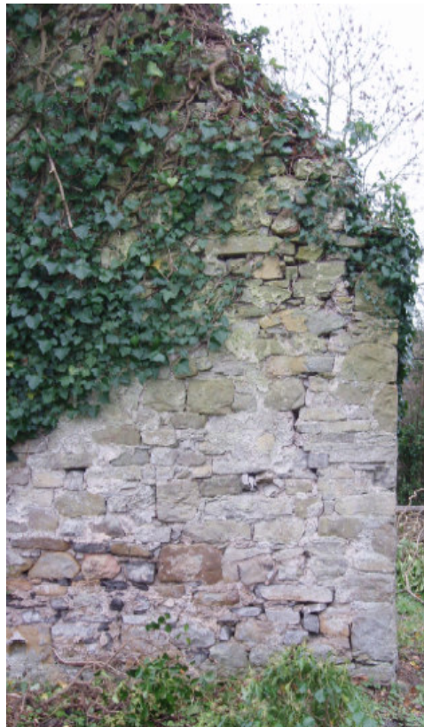
Fig. 17 The south gable end of the east gable also displays movement and needs remedial work
