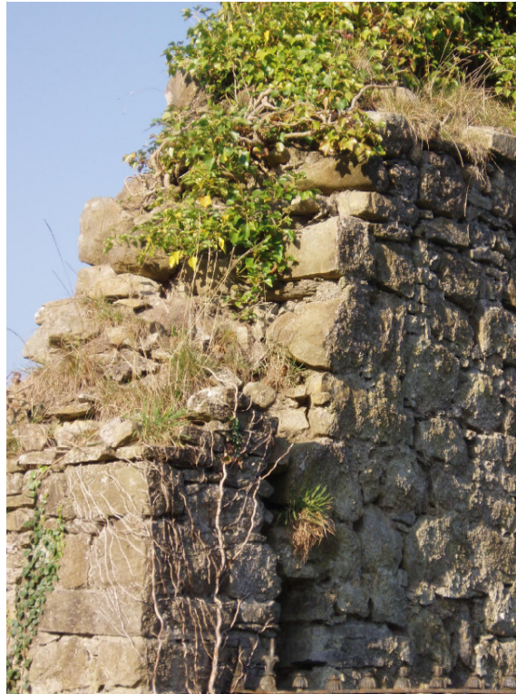
Fig. 9 Ivy and grass have become established on the top of the west gable wall. This should be removed and the masonry conserved
