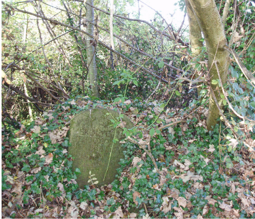
Fig. 36 The south-western boundary wall has collapsed
