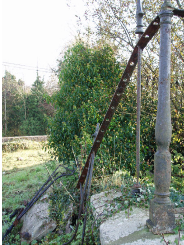
Fig. 35 The north wall of the Singleton plot has collapsed and needs urgent remedial attention
