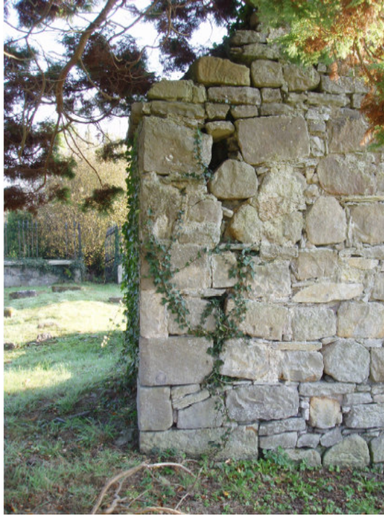
Fig. 11 A large crack and is also apparent at the north end of the west gable. This needs stabilising and conserving
