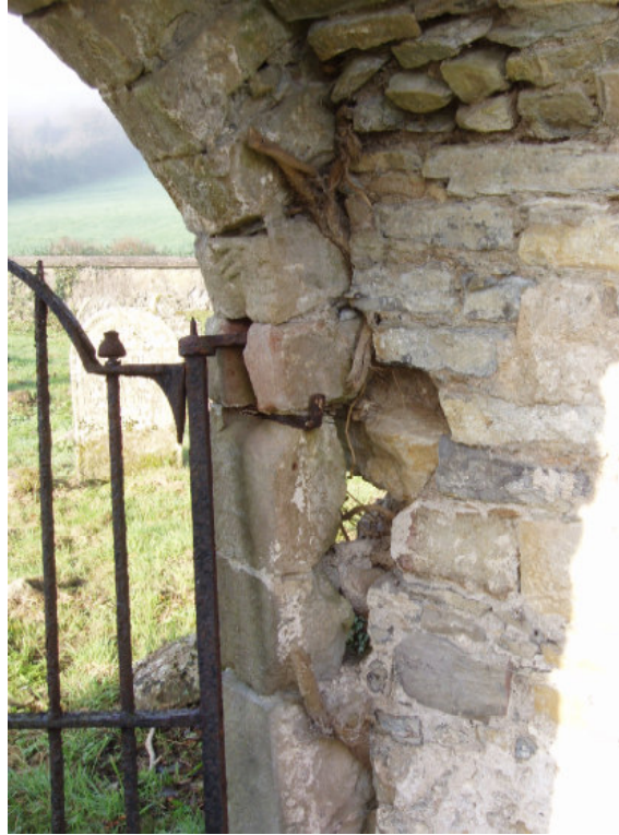
Fig. 12 Detail of the movement in the north jamb of the doorway in the west gable. The gate should be temporarily taken down to enable conservation works to the wall to take place. Once the wall has been consolidated the gate can then be re-hung
