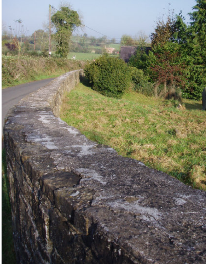
Fig. 39 The coping from the wall is missing and should be replaced
