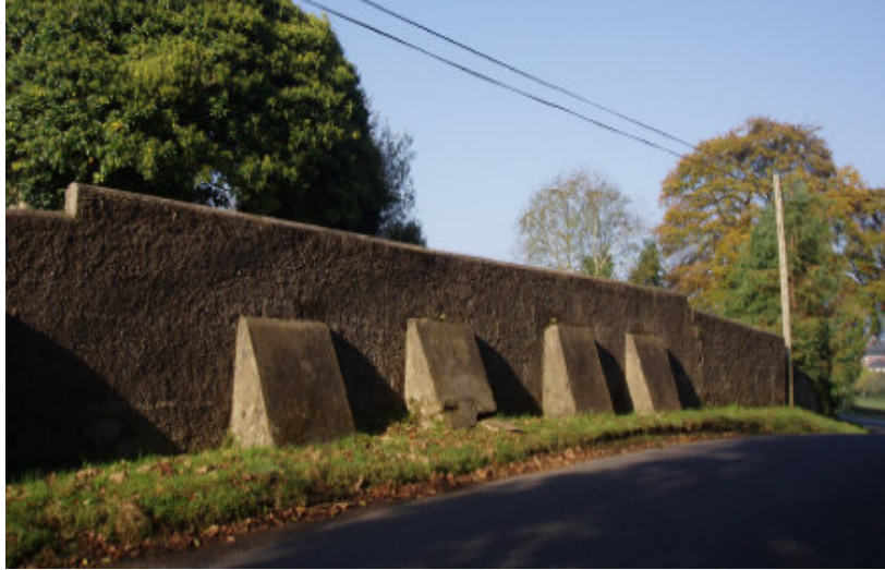
Fig. 41 The east wall of the graveyard has had buttresses added in an effort to retain the wall
