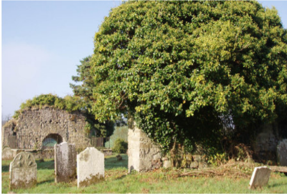
Fig. 16 The east gable of the church is heavily overgrown with ivy
