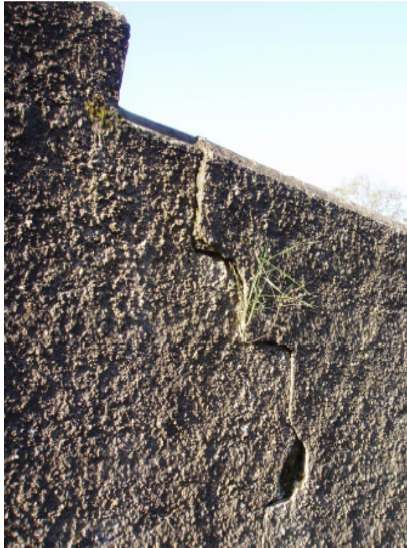
Fig. 43 There is movement in the east wall of the graveyard. The cause of the crack needs to be ascertained to confirm what measures need to be instigated in the future to prevent further damage to the wall. Structural Report on wall recommended
