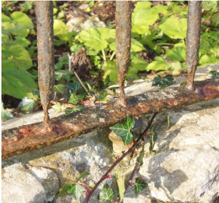
Fig. 30 Detail showing the extent of corrosion to the railings around the Anketell plot
