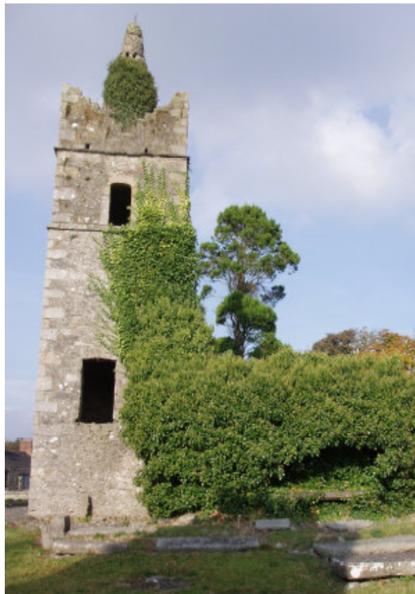
Fig. 12 Ivy covers the south wall of the church and is climbing the tower
