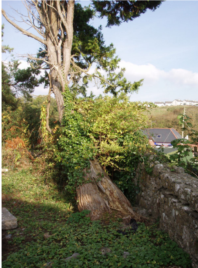
Fig. 22 This yew tree is damaged, and has the potential to destabilise the adjacent wall
