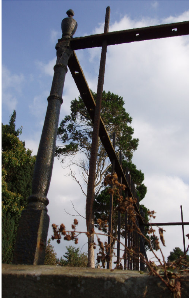
Fig. 30 Some of the railings around the enclosures are missing
