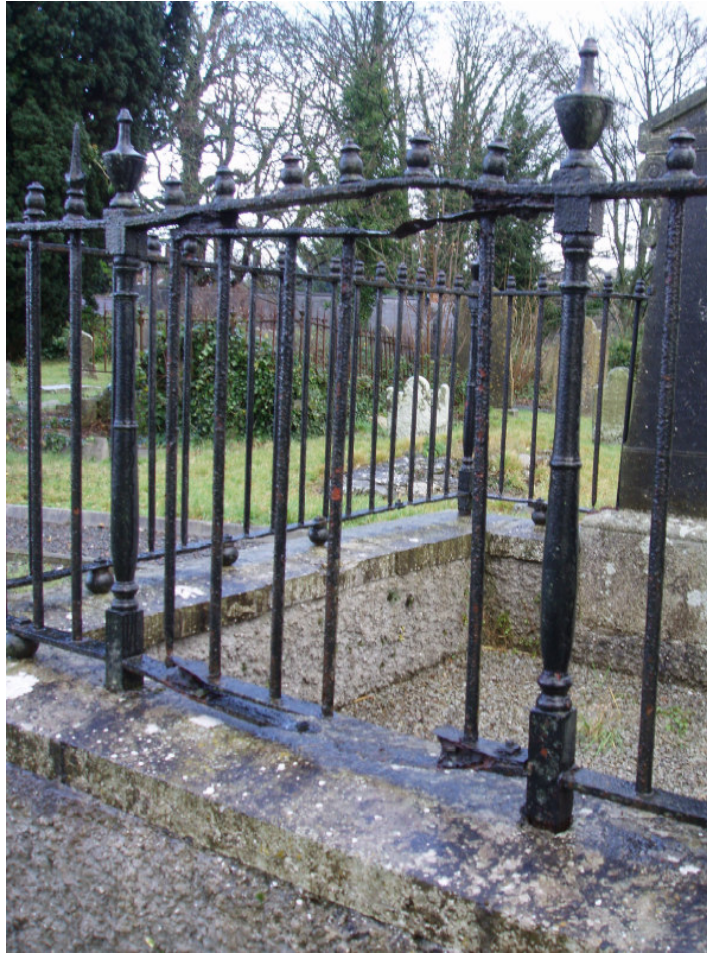
Fig. 38 The gate into Enclosure 5 is in very poor condition
