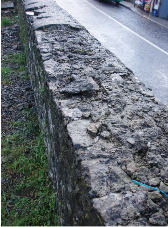
Fig. 45 Parts of the west wall of the graveyard need recapping with a lime-based mortar
