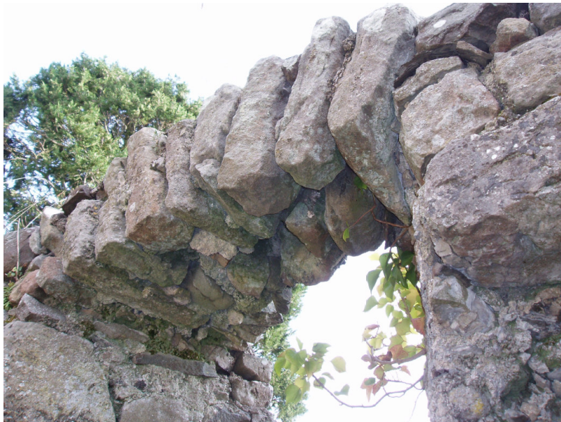
Fig. 14 Detail of the south-east window of the nave, showing the precarious nature of the lintel
