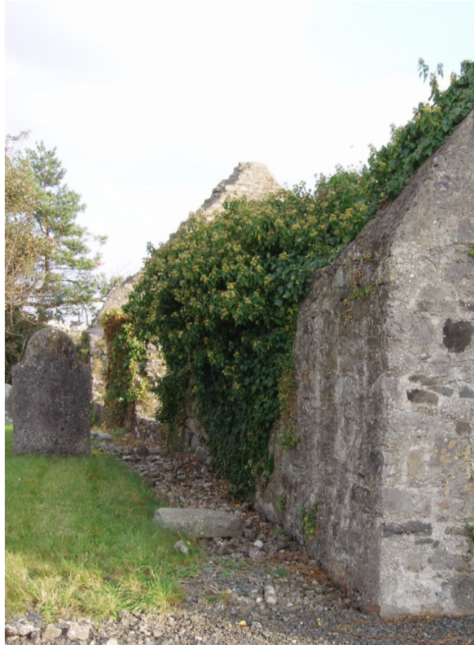
Fig. 19 The north wall of the nave needs its ivy removing
