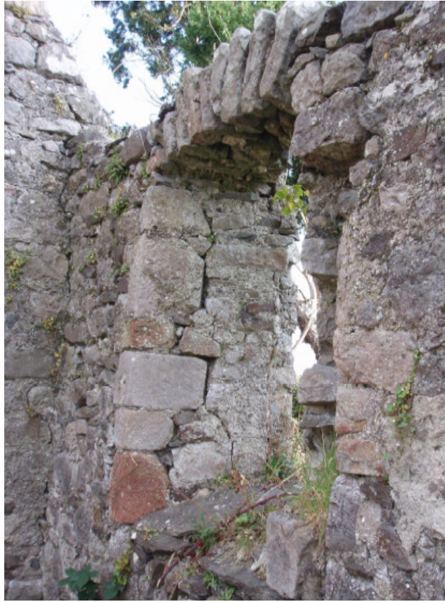
Fig. 15 The south-eastern window in the nave, showing the extent of cracking in the wall
