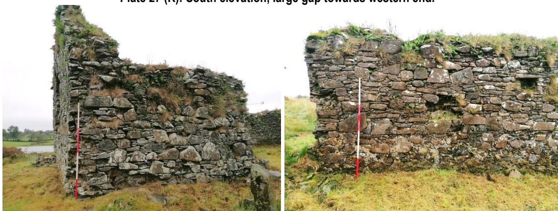
Plate 28 (L): Western side of the south elevation showing the erosion, grass growth and areas of damage and the eroding south western corner.
