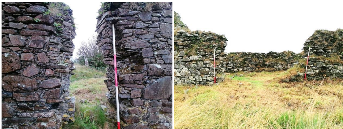
Plate 26 (L): Interior face of south elevation showing narrow collapsed window opening. Note how the stones are placed diagonally to allow for the interior of the window to be wider than the exterior, also note how it appears the window would have sloped upwards to meet in a point.
