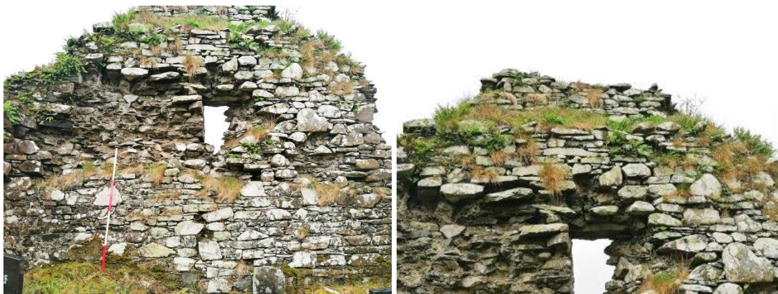
Plate 35: Inner face of west elevation, note the high windows and gaps for corbels, also note the collapse of the centre of the wall Plate 36: Upper part of the wall, Note the grass covered horizontal ledge near the top of the wall for holding the roof rafters
