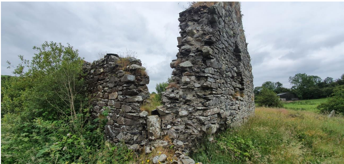
Plate 10: NW corner of Chapel, facing SE, showing collapse and brush overgrowth
