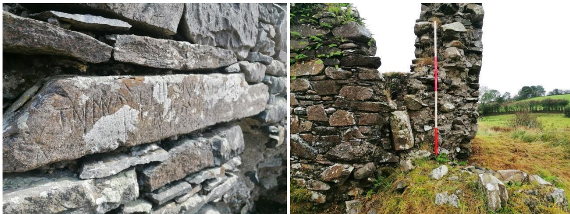
Plate 33: Engraved stone located in NW corner of west gable Plate 34: Collapsed NW corner of the western elevation. Note the heavy westward tilt of the wall
