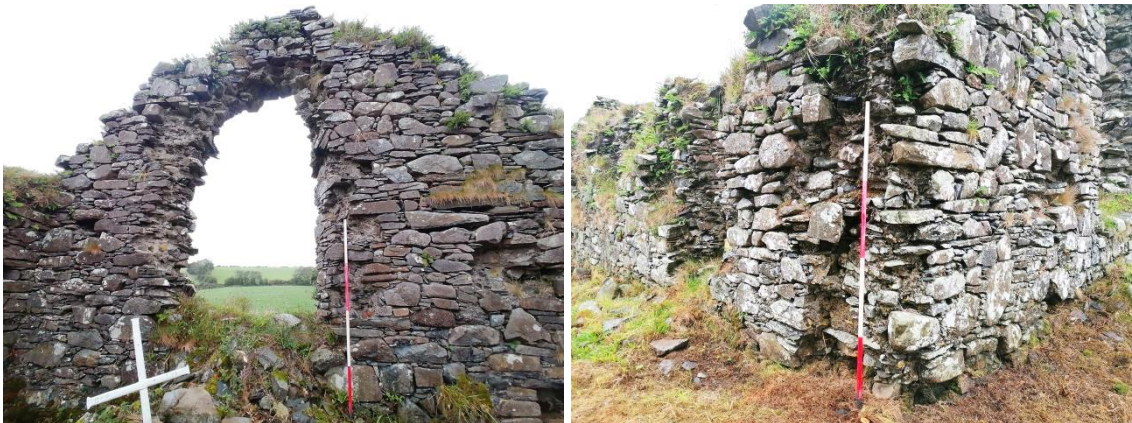
Plate 22 (L): Eastern Elevation (interior), note original window edge and partial arch. Also note the large crack above the opening suggesting the wall is in danger of complete collapse. Plate 23 (R): SE corner collapse, note the exposed mortar
