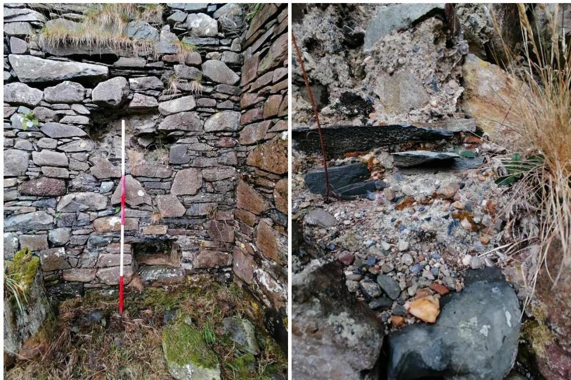
Plate 24 (L): Small box built into the interior face of the Eastern elevation, to the lower southern (right) side. Possibly the ambry, Note areas of collapse and large tree stump (bottom left)
