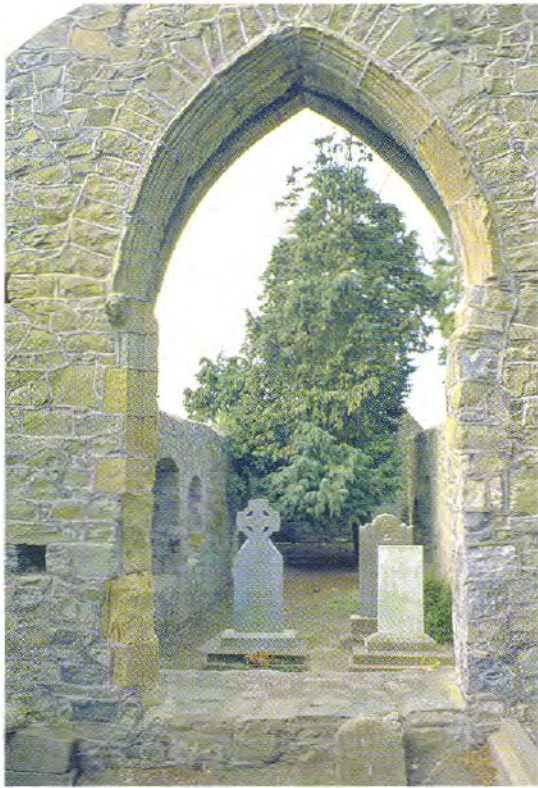
Above The use of cement mortar and ribbon pointing, as shown here, is inappropriate in the conservation of medieval buildings.
