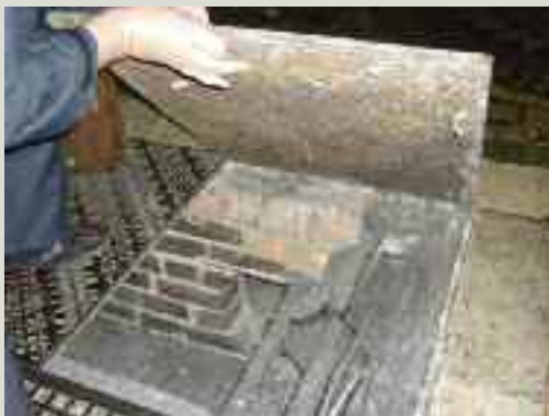
Hot-water heating pipes in a typical nineteenth-century floor duct
