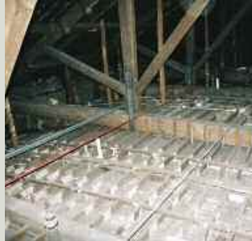
A large roof space with no insulation above the ceiling; while the heat rising from the building interior may benefit the timber and other building materials in the roof space, a lot of energy is wasted in this way
