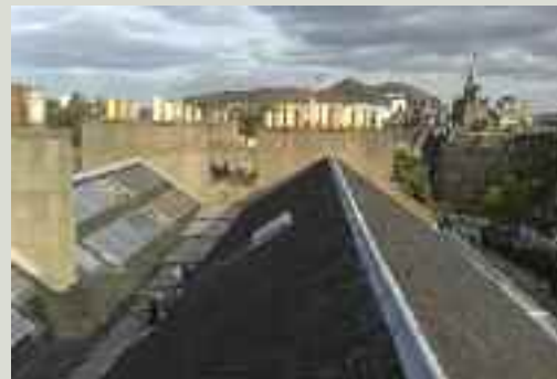
A roof valley may be an appropriate place to locate solar thermal or photovoltaic panels provided that the orientation of the roof is appropriate. This image shows solar panels installed in hidden roof valley as part of Changeworks' Renewable Heritage project (Image © Changeworks)
