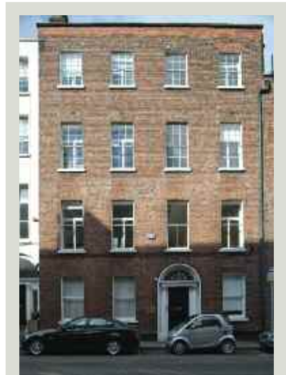
Inappropriate timber-framed secondary glazing with frame proportions that do not match those of the original window, creating a discordant appearance
