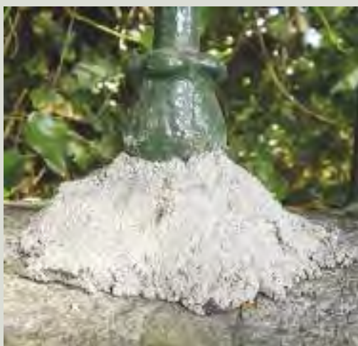
Concrete is not an appropriate material for the repair of ironwork, particularly in combination with stone
