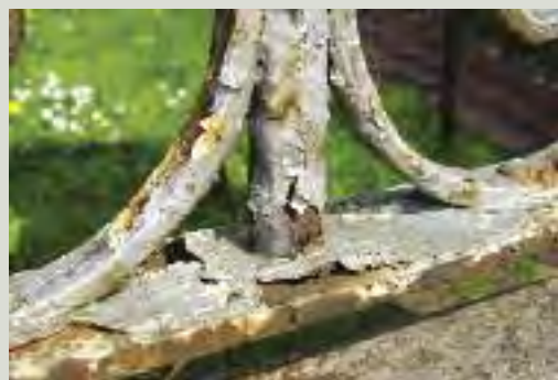
Broken, flaking paint traps and holds water to the iron, preventing it from drying out properly, and can lead to corrosion. Areas of chipped paint are not as significant a threat so long as the iron is in an exposed location and is able to dry out. Nevertheless, such chips should be treated as soon as possible to prevent rust from forming
