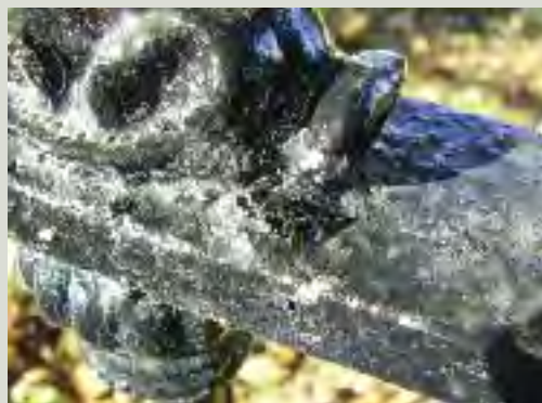
This photograph shows a set of railings a month after they were painted. Corrosion material was not thoroughly removed before the application of paint resulting in the localised failure of the new paint
