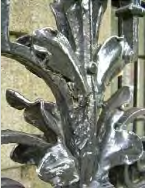
Water traps, such as the void areas behind these leaf details, will cause corrosion to develop at a faster rate
