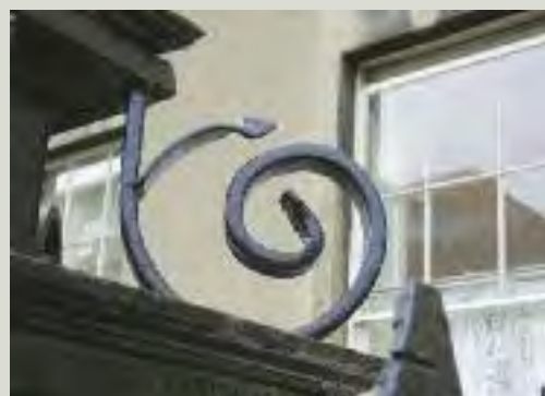
It is important to choose an experienced craftsman to avoid inappropriate repairs. The replacement scroll in the lower image has been crudely formed and bears little resemblance to the finely-crafted original feature on a neighbouring property in the top image
