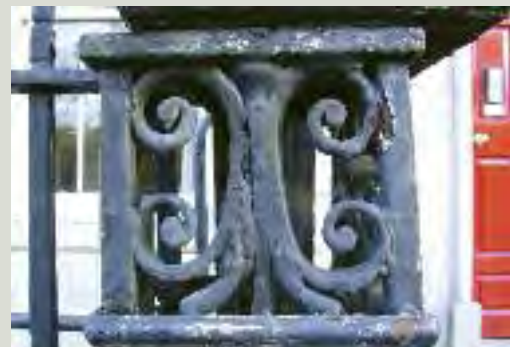
Posts from two different properties on Parnell Square, Dublin. While appearing to be severely corroded, much of the original ironwork in the lower example may remain intact beneath layers of paint and corrosion
