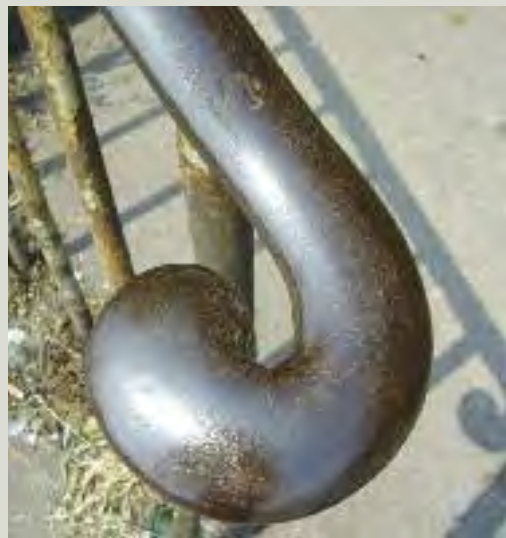
An oxide layer has developed on this wrought iron handrail which protects it from further corrosion
