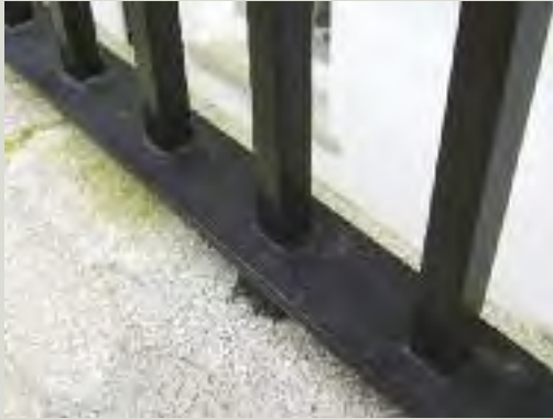
Replacement bars should pierce through the rail rather than be welded to it (as shown above)
