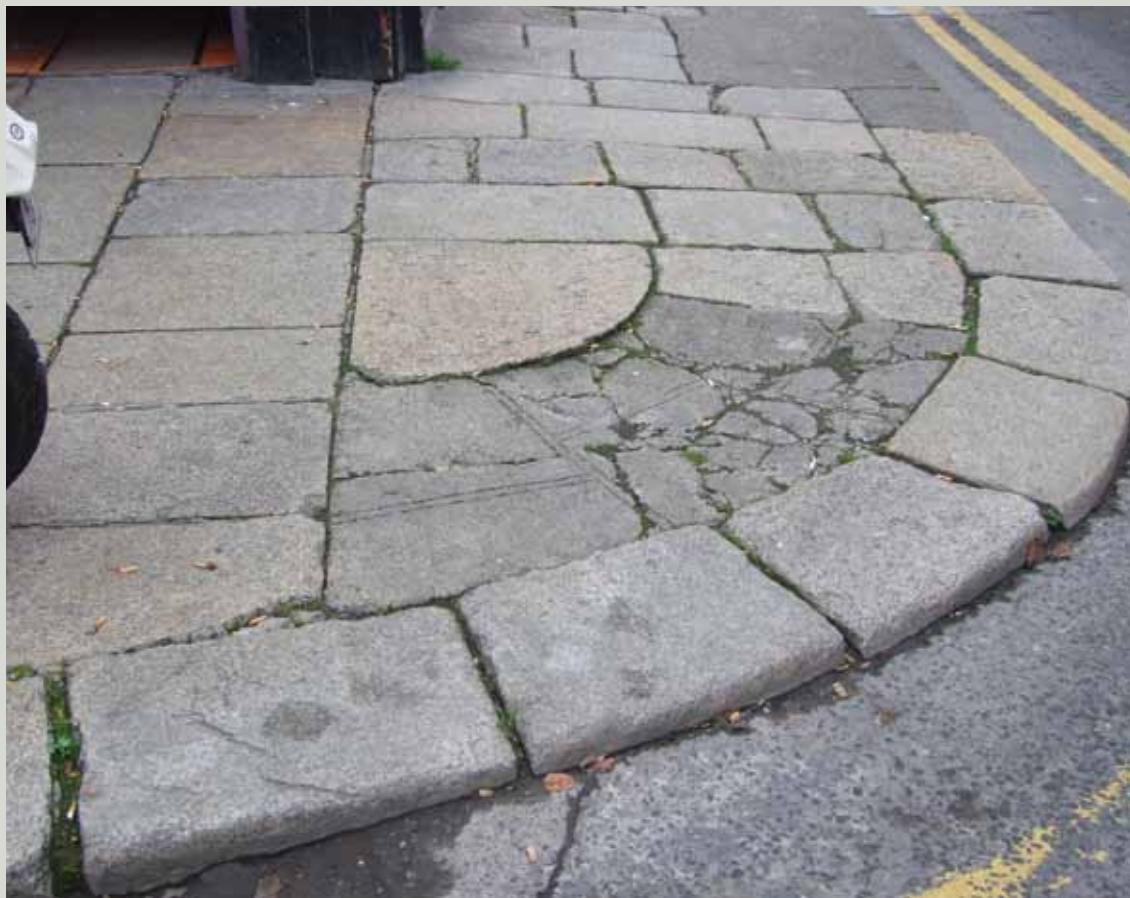
The repair of this radial corner will be labour-intensive work and require particular skill to repair correctly
