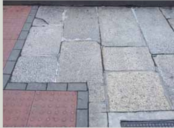
New inserts should follow the layout of the historic flags and not require the cutting of the existing stones as has happened in this case
