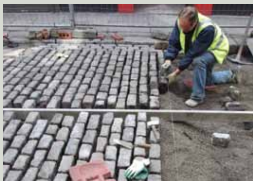
Sett-laying in rigid construction without contact between setts. Note inconsistent joint width which is a result of the setts not having been sorted according to size.
