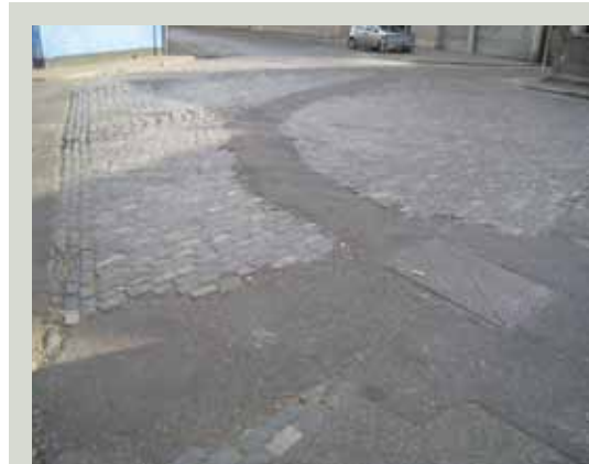
Extensive damage to a setted pavement caused by laying of underground services
