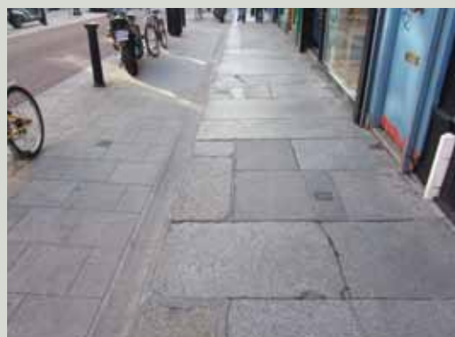
A widened pavement has left the original flags in situ while constructing the new section in a compatible material. The final appearance would have been improved if the sizes and pattern of the new and old flags also matched and the joint between old and new was tighter and filled with a more appropriate pointing material
