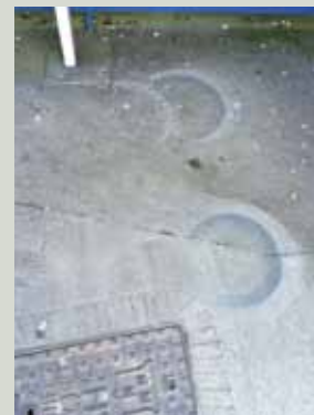
Damage from mechanical cleaning equipment can be seen on this concrete pavement
