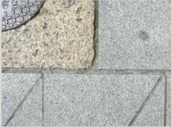
Inappropriate sawn stone edges and sharp corners, in addition to poor colour matching, give a discordant appearance against the texture and softened edges of the historic granite
