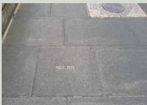
Significant details should be recorded such as this example of the manufacturer's name inlaid in brass into a concrete flagstone
