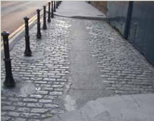
A historic surface has been damaged by poor workmanship in erecting bollards to prevent parking and in laying underground utilities, leading to unnecessary loss and damage of setts
