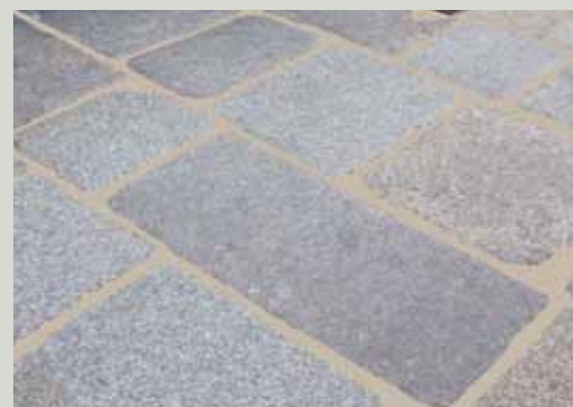
These images show the effects of different pointing methods on the same area of paving; in the top image the joints are recessed, while in the bottom one the joints are flush, or marginally recessed, using a light-coloured mortar
