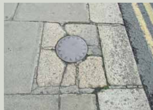
Damaged granite flagstone surround to a coalhole cover. However, despite the damage it should be retained in situ with whatever minor repairs are required to mitigate further damage
