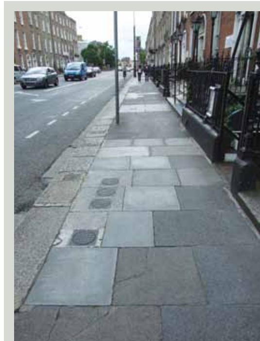
Access covers installed along a highly significant Georgian street have created a patchwork of different materials and flagstone sizes which disrupt the appearance of the Neo-classical street
