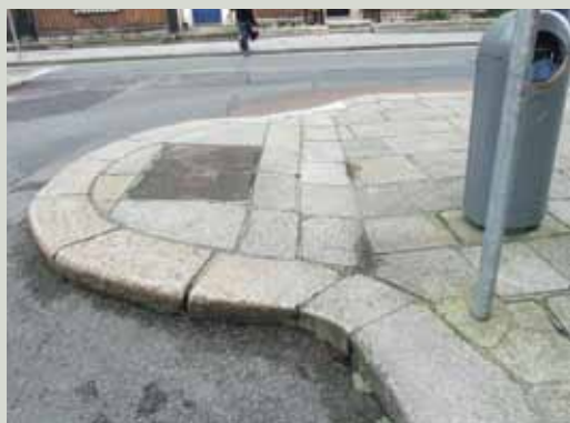
Historic flagstones and kerbs re-laid in an incongruous modern layout
