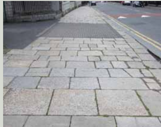
Modern brick panels inserted into historic paving help to avoid damage and cracking of granite flagstones by heavy vehicles driving over. However, the use of modern engineering brick is visually unsatisfactory
