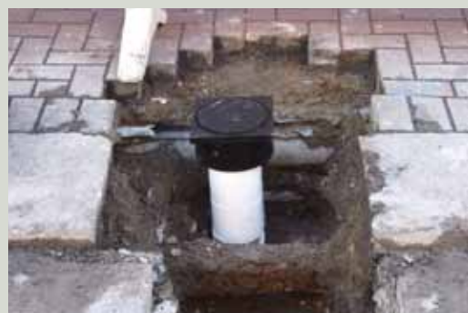
The granite kerb has been cut through and partially lost rather than locating the new installation within the area of modern paving
