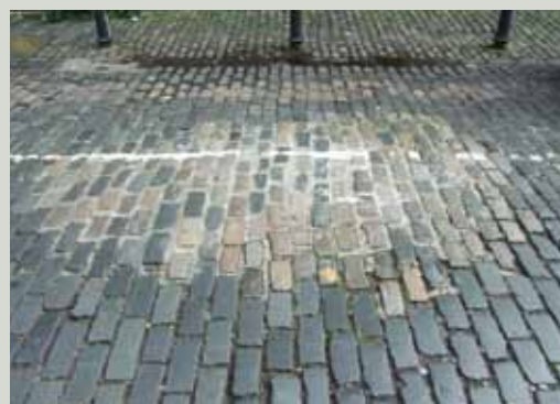
Unsuccessful repair using setts of different stone types, poorly set out and using inappropriate jointing material and methods
