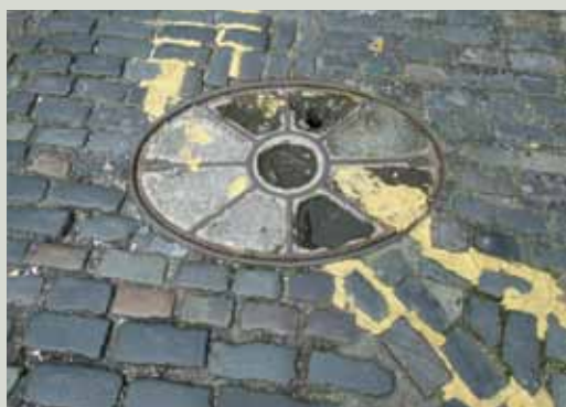
Oval cover originally with timber inserts which have been inappropriately replaced with cement
