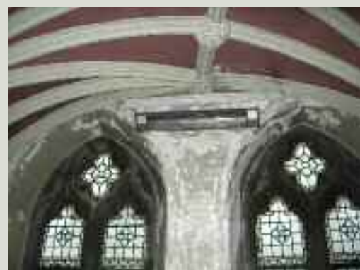
Church lighting and heating systems may evolve on an ad-hoc basis as funds become available. In this case, strip lights and electric bar heaters were fitted to some of the aisles. Conservation works to the church will include the removal of these fittings and repairs to the roof above to eradicate the damp in the wall
