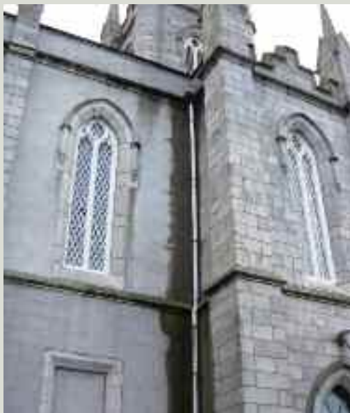
Walls will quickly become saturated if rainwater cannot be shed effectively from the roof. Staining, discolouration and plant growth behind and beside downpipes are signs of problems at eaves or parapet level that require immediate attention
