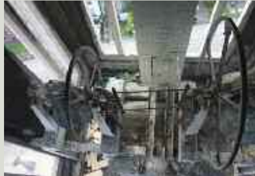
This belfry was photographed prior to work commencing on the steeple (but after the louvres were removed to provide more light for the duration of the project). In common with all such areas, the signs of pigeon infestation are everywhere, however the structure and bell mechanism are in a reasonable condition
