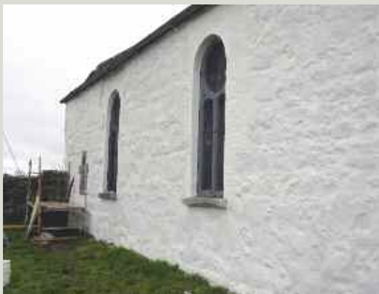
The rubble walls on this medieval parish church were stripped of roughcast cement render and re-rendered using a soft lime mortar. This helped the interior of the building to dry out, assisting to preserve the significant Romanesque stone carving
