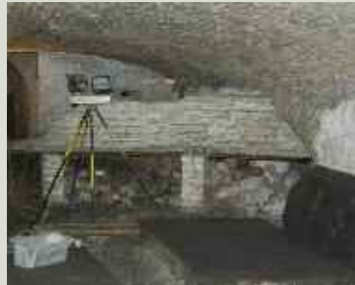
Inspecting a crypt presents risks such as trip hazards, toxic fumes, asbestos and rodent or fungal infestation. Personal protective equipment and adequate lighting are essential to reduce the risk of accident to the inspector or damage to the structure
