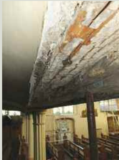
Regular inspections and scheduled maintenance work should prevent rot from taking hold to the degree that it causes structural damage, as has happened to this beam which supports an organ gallery
