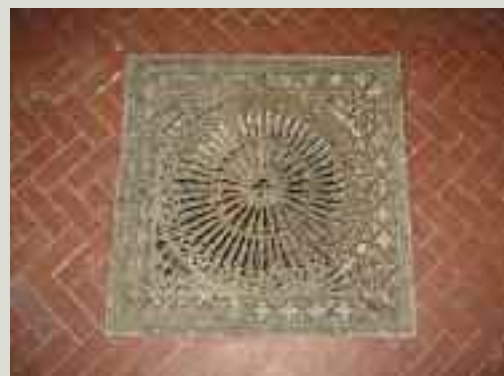
Several elements of a historic heating system often survive, as at this church where both boiler and perforated floor grilles remain
