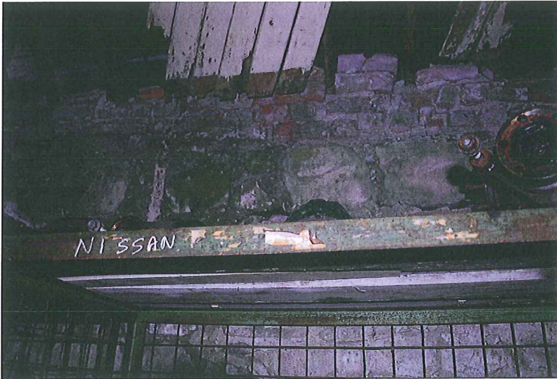
Side elevation (south) interior, with original beam to ceiling. Four courses of redbrick above stone.
