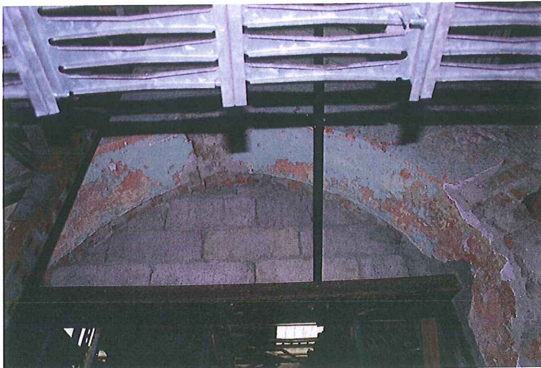
Former window on back gable wall, now forms door access to workshop.
