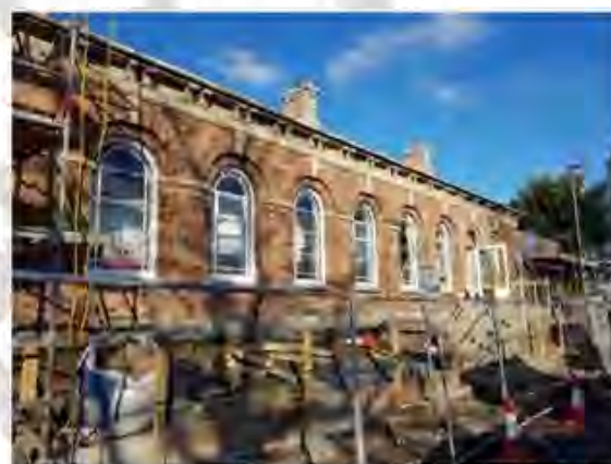
New windows installed in Station Master's House with built heritage funding to reflect the openings of the recently restored Railway Station building adjacent
