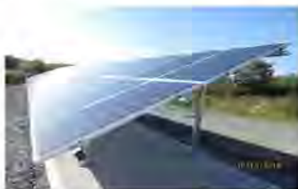
Photo of Solar PV Installation – Scotch Corner
