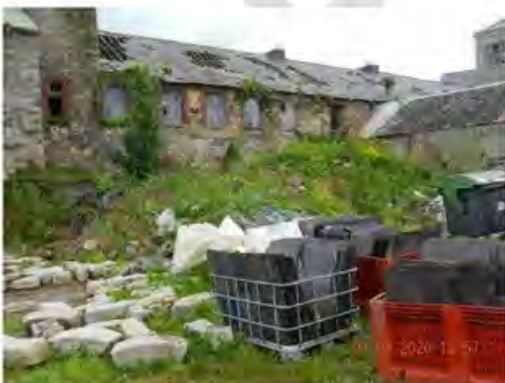
Roof of rear Carrickmacross Workhouse building partially collapsed and dangerous
