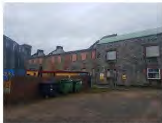
Carrickmacross Workhouse windows have been shored and boarded up and damaged elements of the roof structure removed
