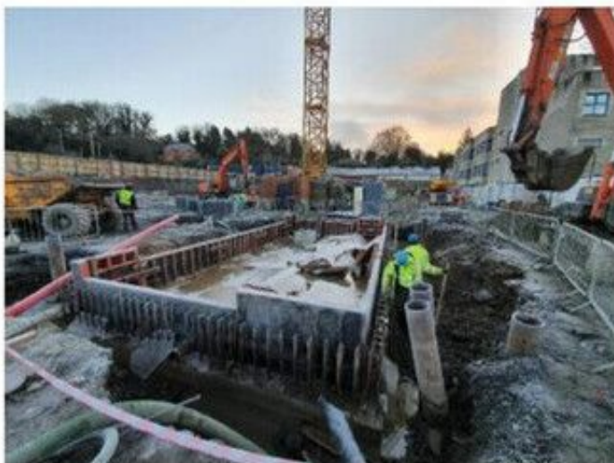
Attenuation tank nr2- Rebar and formwork white with frost, backfilling of base ongoing
