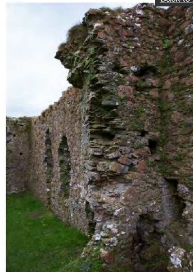
Vulnerable section of wall west of the Great Hall
