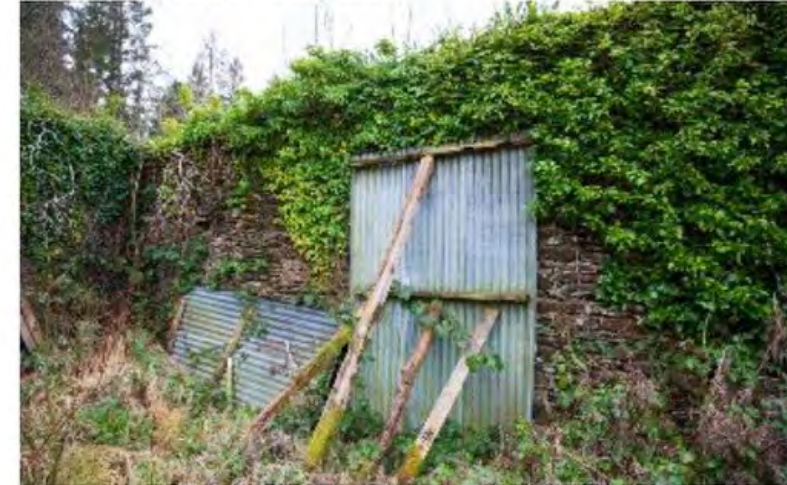
A blocked entrance and overgrown section of wall
