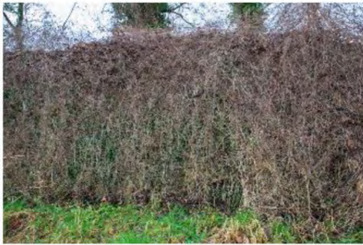
An overgrown section of wall
