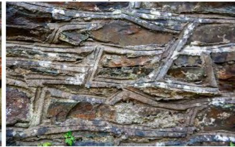
Concrete used as mortar – this causes great damage as the concrete is not breathable
