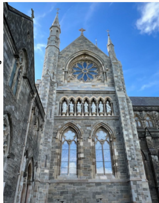
Fig. 3: Conservation works to the external and internal facades of the north transept gable at St. Macartan's Cathedral, Monaghan
