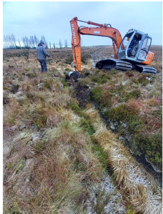
Creating a peat dam to block drain on Sliabh Beagh to restore the hydrological functions of the blanket bog.
