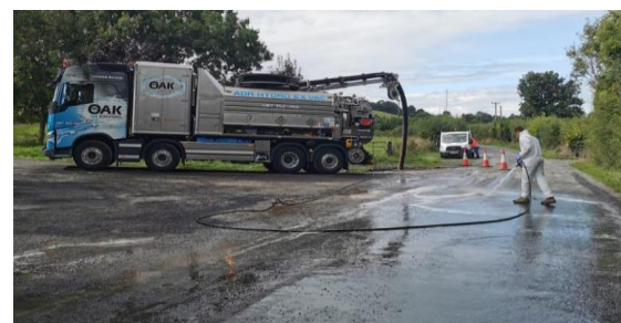
Diesel wash Clean-up in Donaghmoyne
