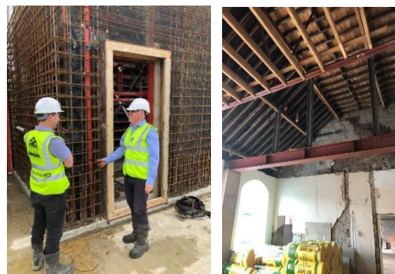
Building Control inspections of Peace Campus and HSE Blackwater House facility in Monaghan June 2022
