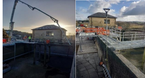
Ballybay WWTP under IWSS Programme
