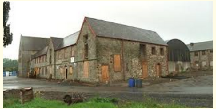
Rear Derelict Buildings
