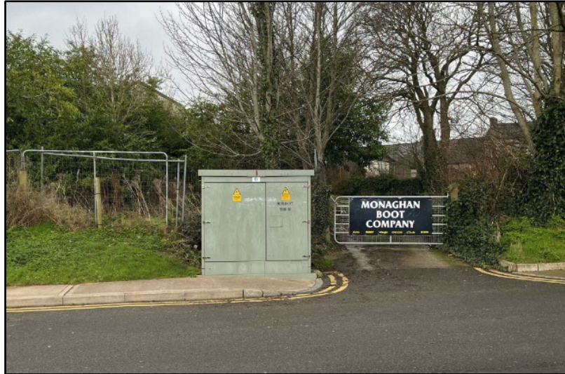
Figure 2.34: Existing ESB sub station
