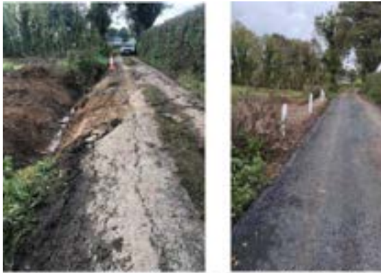
Figure 3 & 3 : Pre and Post work photos of verge (Appage) repairs on the L73-4203 at Garraun
