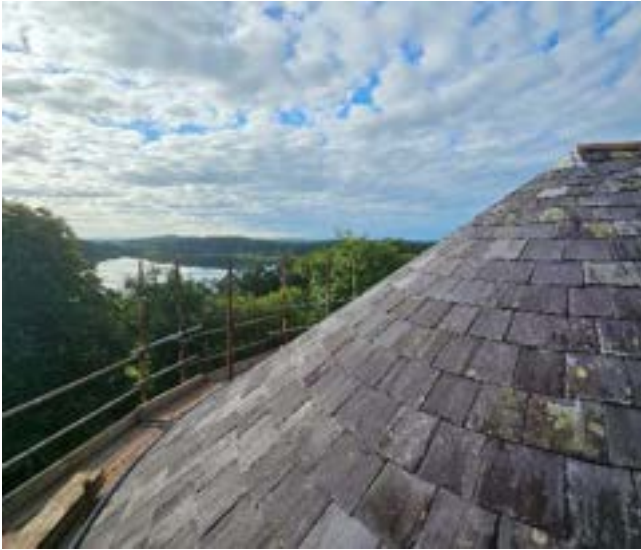
Completed conservation work to the roof at St. John the Evangelist Church, Dartrey
