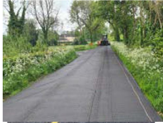
Figure 10: Resurfacing Improvement Grant, Surface Dressing strengthening works of the R-662 at Killybegs
