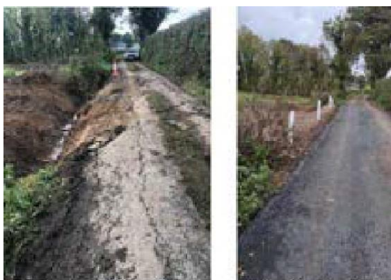
Figures 2 & 3 | Pre and Post work photos of ramps (Average repairs on the L704200 at Garraí)
