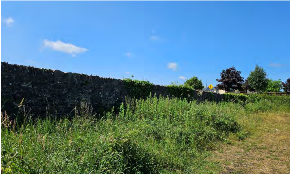
Wing wall to bridge to the east of the bridge adjacent to the proposed hardstanding.
