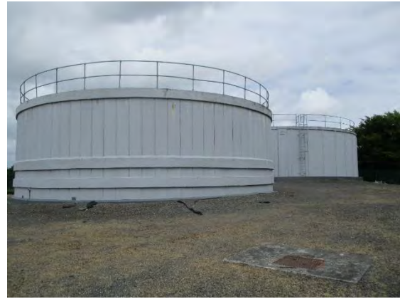
Corduff/Corracharra GWS Treated Water Reservoirs, Reservoirs are in need of repair and have been added to the MARWP 2024-2026
