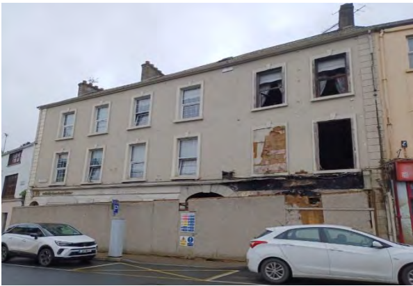
24-26 Market Street. Property was fire damaged in 2017. MCC have progressed towards Compulsory Purchase Order proceedings
