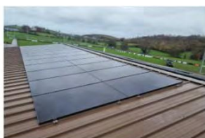
Traugh Gaeils GFC- Solar PV System
