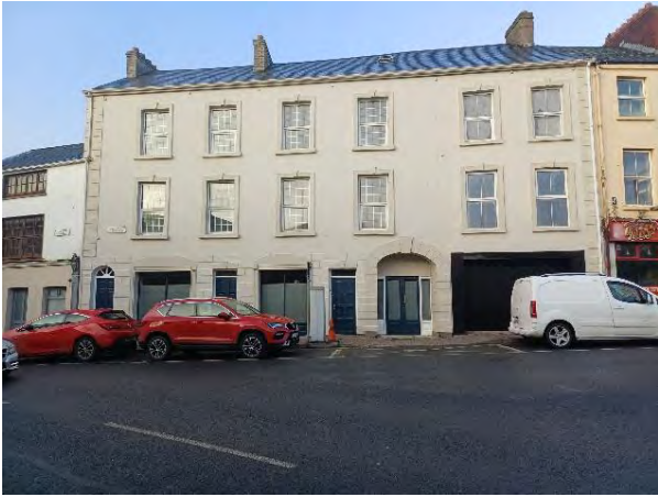
24-26 Market Street. Property was fire damaged in 2017. MCC started CPO proceedings, but property was sold to developer who has started to undertake works
