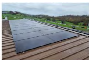
Traugh Gaeils GFC- Solar PV System
